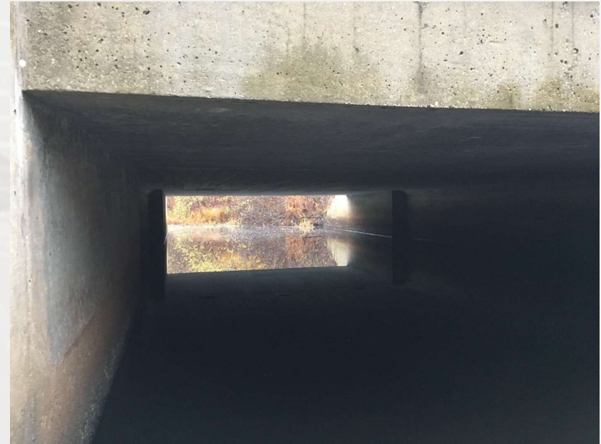
Laitance at Widening Joint
