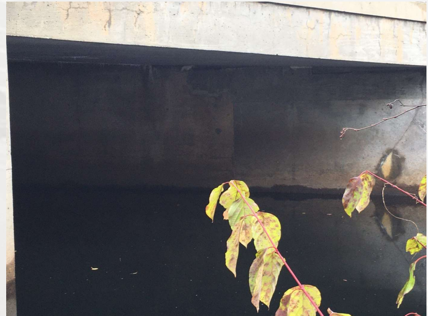
Laitance at Widening Joint
