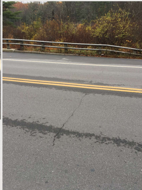
Transverse Cracks in Pavement
