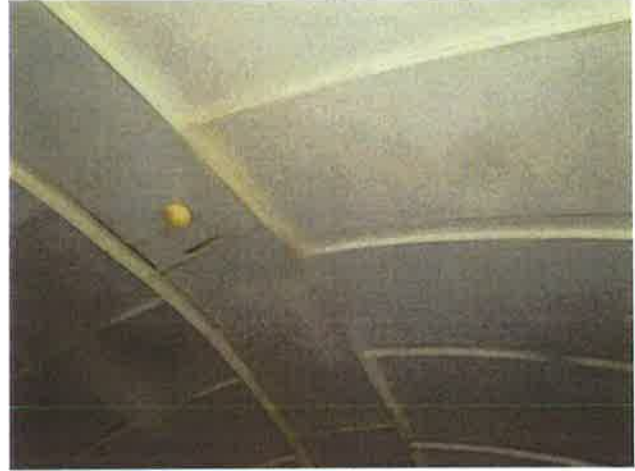
88 Overhead With Mild Blotch Rusting
