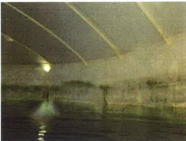
83 Interior Wall With Moderate To Heavy Staining
