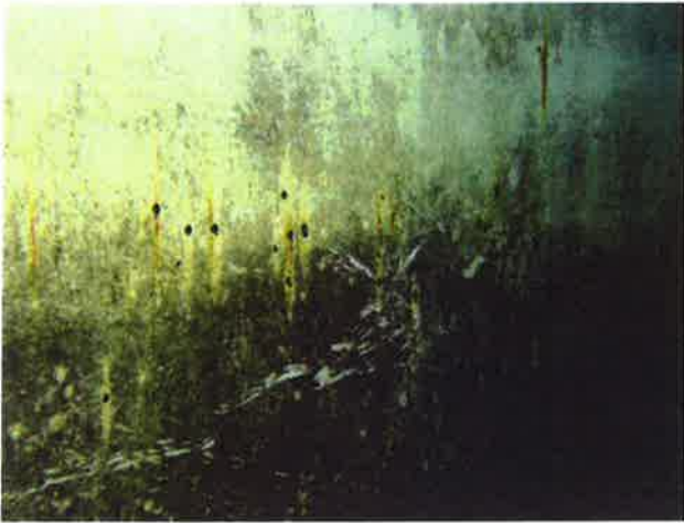
67 Interior Wall With Coating Loss, Exposed Steel, Surface Corrosion And Moderate To Heavy Staining
