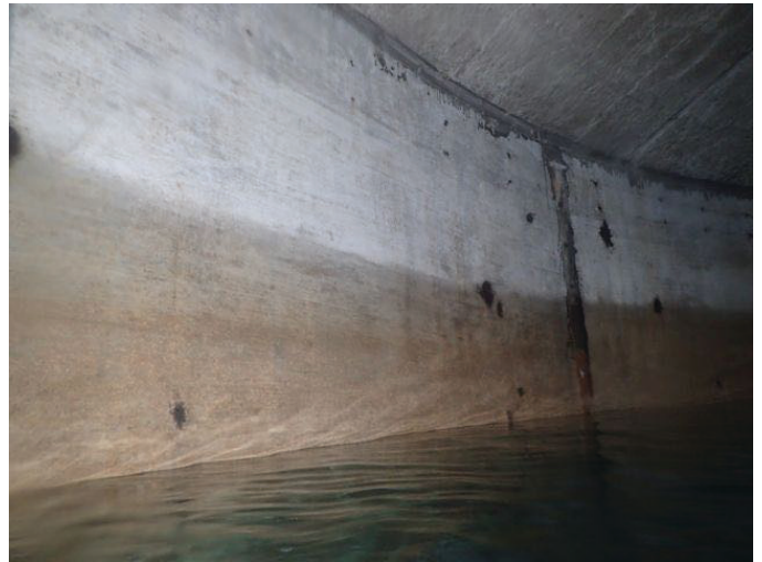
70 Interior Wall With Mild Staining
