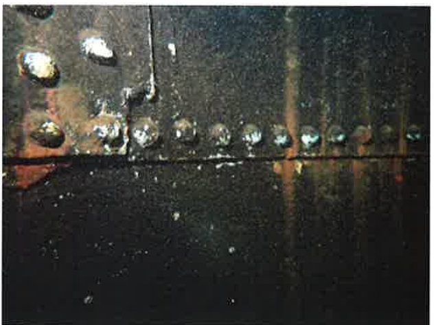
66 Interior Wall With Coating Loss (Nearing Expiration), Blotch Rusting, Exposed Underlying Steel, Moderate Surface Corrosion And Heavy Staining
