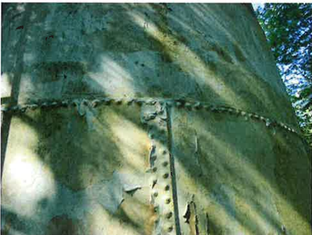
5 Exterior Wall With Expired Coating/Peeling, Exposed Underlying Steel, Blotch Rusting, Mild To Moderate Surface Corrosion, Corrosive Staining, Rust Staining And Mildew
