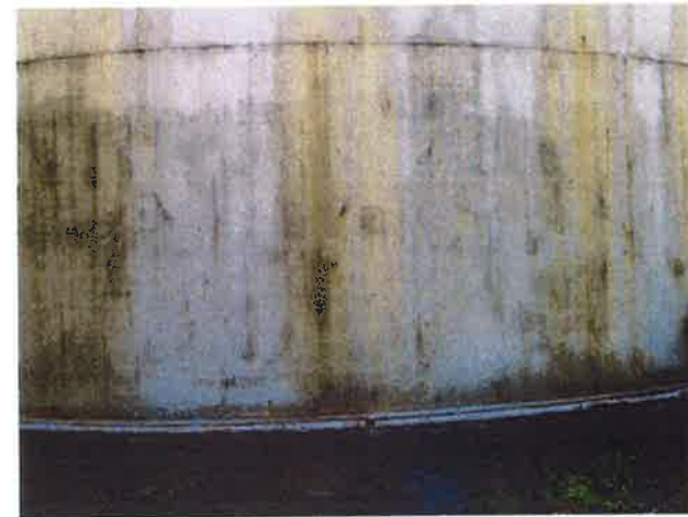
6 Exterior Wall With Coating Loss/Damage, Chalking Exposed Underlying Steel, Mild Surface Corrosion, Mildew And Corrosion Staining
