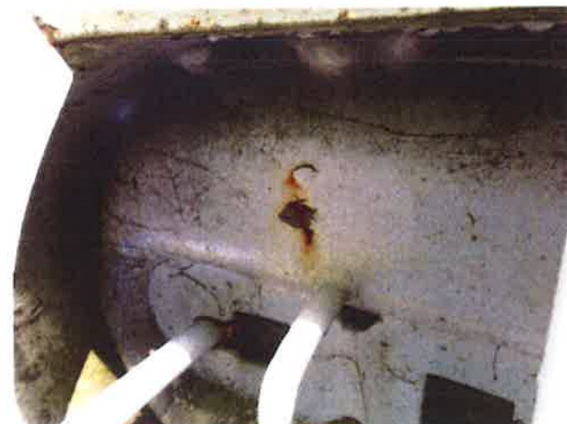
18 Manway Lid With Coating Loss, Exposed Steel And Mild Surface Corrosion
