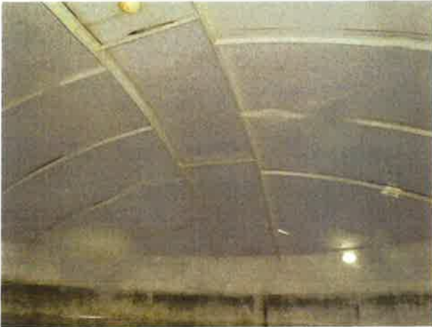
87 Overhead With Mild Blotch Rusting
