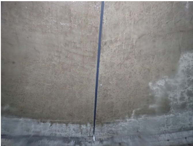
81 Overhead With Panel Joints/Edges With Efflorescence
