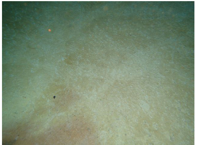
38 Floor With Mild Staining
