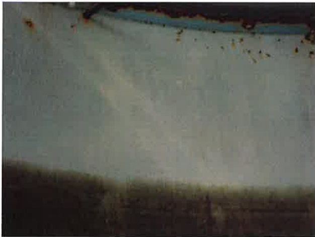
75 Interior Wall With Ruptured Coating Blisters, Exposed Underlying Steel, Mild To Moderate Surface Corrosion And Heavy Staining
