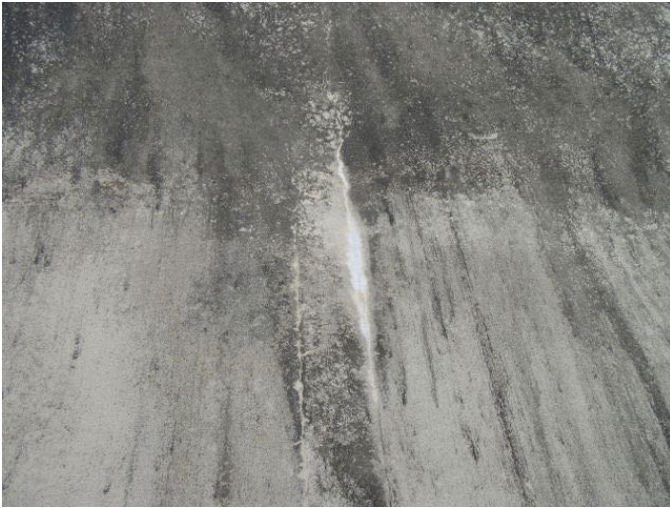
21 Roof Dome Concrete Filled Joints With Coating Loss, Tight Cracks And Mildew
