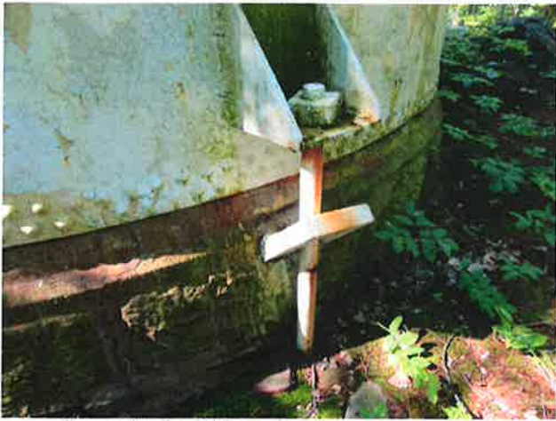
31 Secure Anchor Bolt With Coating Loss
