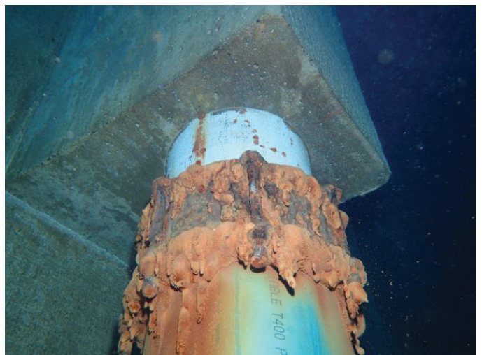
54 12" Inside Diameter P.V.C. Piping Extending Through A Coupling And Penetrating A Concrete Box With Coating Loss/Blistering, Exposed Metal And Corrosion
