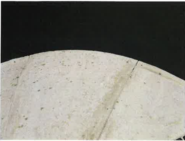
37 Roof Panel Joints Sealant Found Deteriorating
