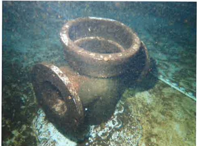
58 T-Fitting Inlet/Outlet Pipe Penetrating The Tank Floor
