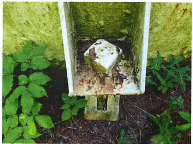
32 Secure Anchor Bolt With Coating Loss
