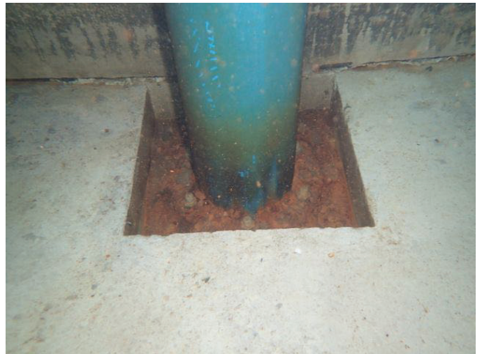
82 Overflow Pipe Penetrating The Tank Floor Within A Deep Sump
