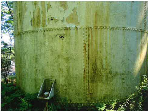
3 Exterior Wall With Expired Coating/Peeling, Exposed Underlying Primary Coating, Rust Staining And Mildew
