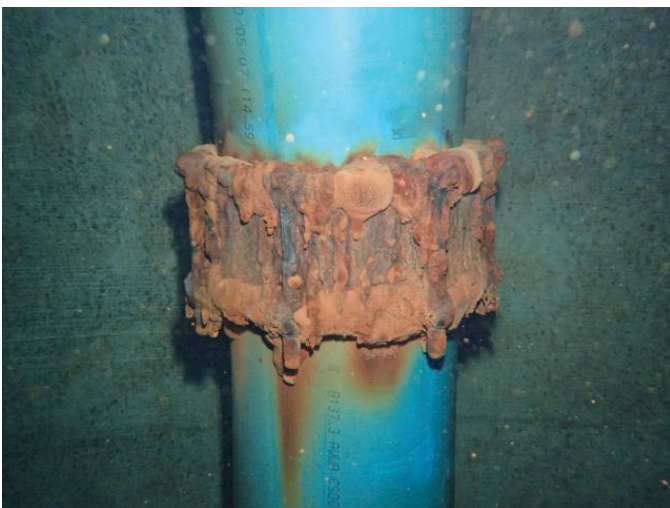
53 12" Inside Diameter P.V.C. Piping Extending Through A Coupling With Coating Loss/Blistering, Exposed Metal And Corrosion
