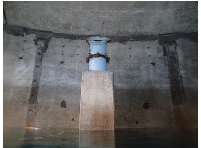
56 12" Inside Diameter And Elbow Extending From The Top Of The Concrete Box
