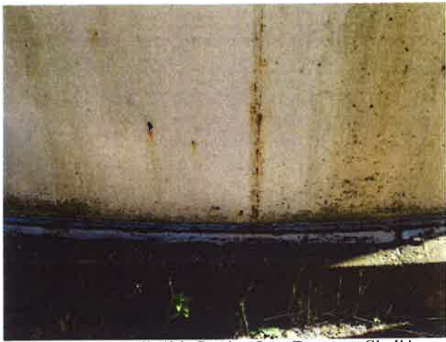
1 Exterior Wall With Coating Loss/Damage, Chalking Exposed Underlying Steel, Mild Surface Corrosion, Mildew And Corrosion Staining
