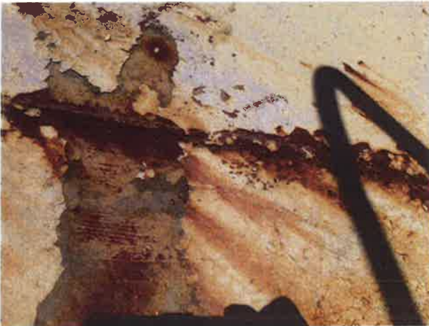
33 Roof With Coating Nearing Expiration, Exposed Primary Coating, Exposed Underlying Steel, Mild Surface Corrosion And Corrosion Staining
