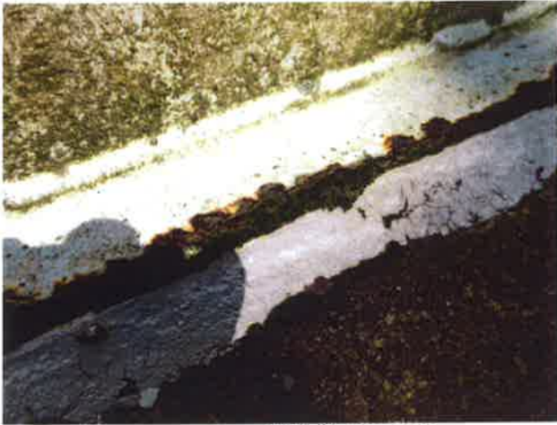
13 Steel Floor Extension With Coating Loss, Exposed Steel, Mild To Moderate Surface Corrosion And Mildew
