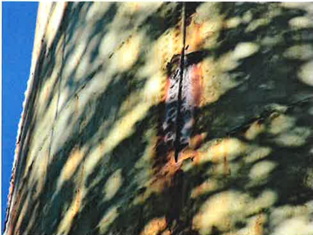
15 Exterior Wall With Expired Coating/Peeling, Exposed Underlying Steel, Blotch Rusting, Mild To Moderate Surface Corrosion, Corrosive Staining, Rust Staining And Mildew
