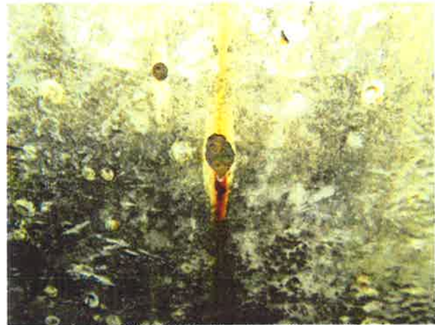
58 Interior Wall With Coating Loss, Exposed Steel, Surface Corrosion And Moderate To Heavy Staining
