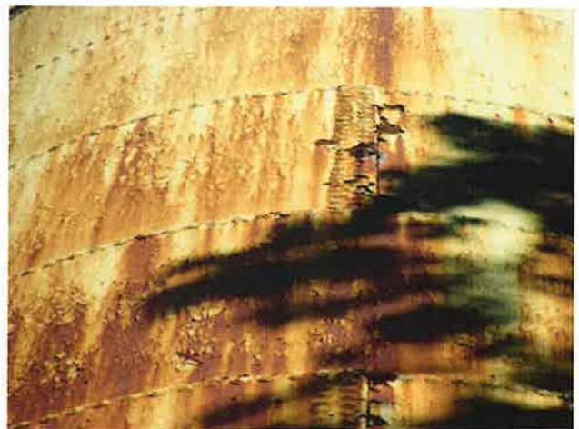
12 Exterior Wall With Expired Coating/Peeling, Exposed Underlying Steel, Blotch Rusting, Mild To Moderate Surface Corrosion, Corrosive Staining, Rust Staining And Mildew
