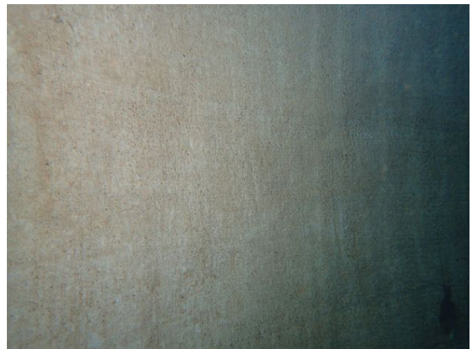
66 Interior Wall With Mild Staining
