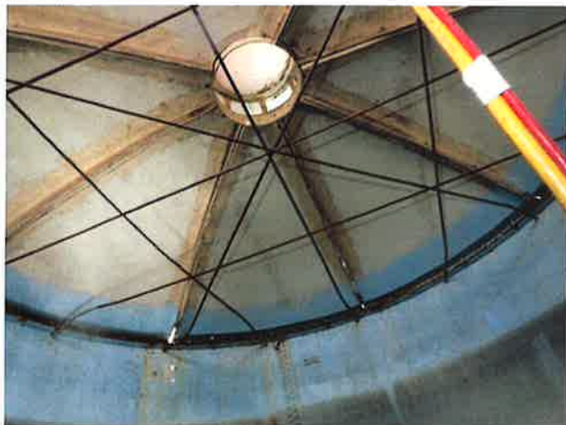
81 Overhead Spider Supports With Mild Surface Corrosion
