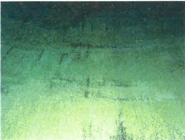
77 Interior Wall With Moderate To Heavy Staining
