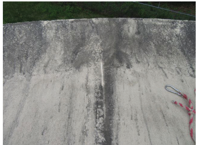
24 Roof Dome Concrete Filled Joints With Coating Loss, Tight Cracks And Mildew
