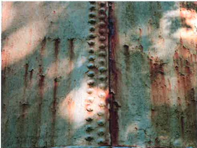
21 Exterior Wall Third Row Vertical Lap Joint (East Side) Found Appearing Damp And Moist
