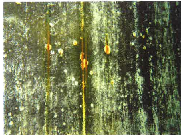
60 Interior Wall With Coating Loss, Exposed Steel, Surface Corrosion And Moderate To Heavy Staining
