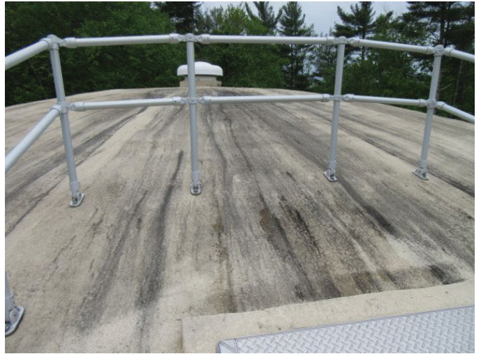
26 Secure Safety Railing
