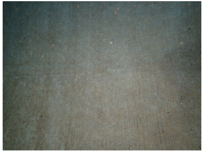
64 Interior Wall With Mild Staining
