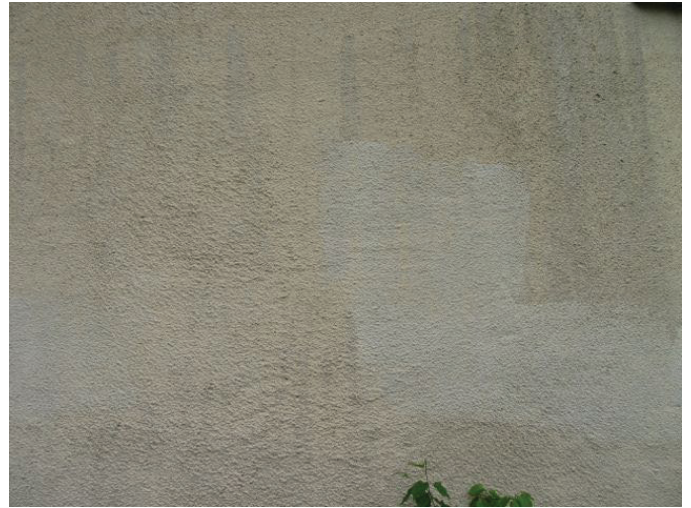
8 Exterior Wall With Mild Mildew
