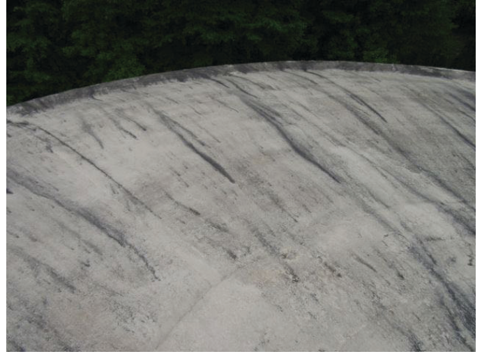
20 Roof Dome Concrete Filled Joints With Coating Loss, Tight Cracks And Mildew
