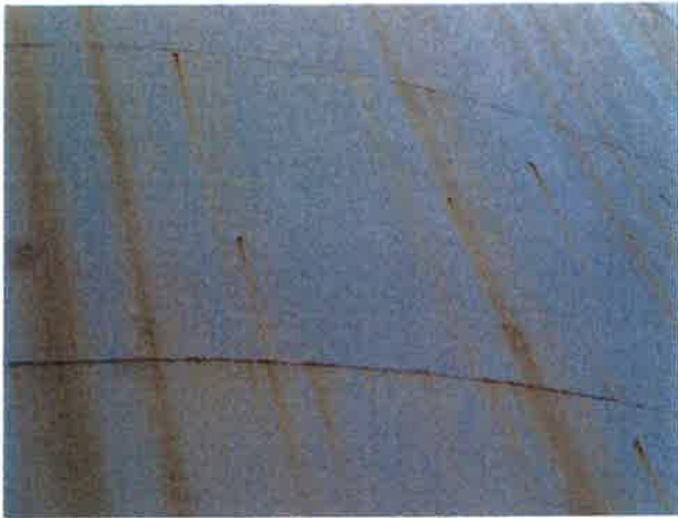
7 Exterior Wall With Coating Loss/Damage, Chalking Exposed Underlying Steel, Mild Surface Corrosion, Mildew And Corrosion Staining
