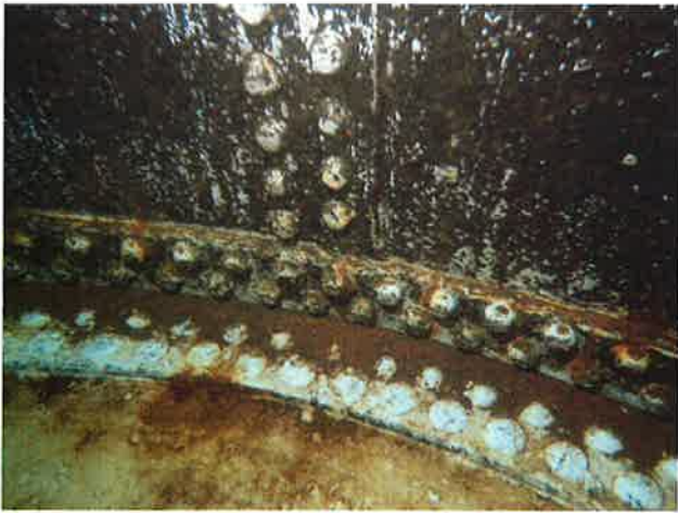
61 Interior Wall With Coating Loss (Nearing Expiration), Blotch Rusting, Exposed Underlying Steel, Moderate Surface Corrosion And Heavy Staining
