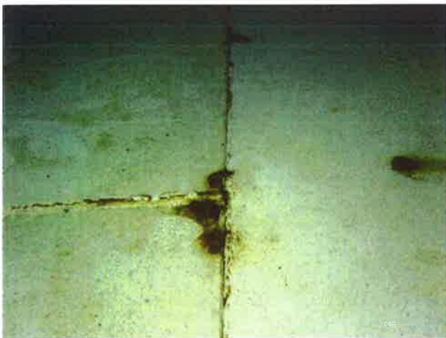
47 Floor With Ruptured Coating Blisters, Exposed Underlying Steel, Mild Surface Corrosion And Mild Staining
