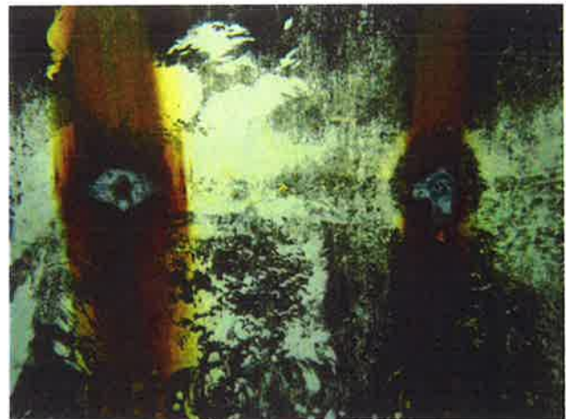
72 Interior Wall Welds With Coating Loss, Steel Fatigue (Pitting) And Moderate To Heavy Staining
