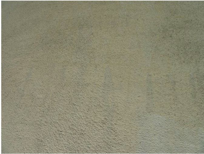
7 Exterior Wall With Mild Mildew
