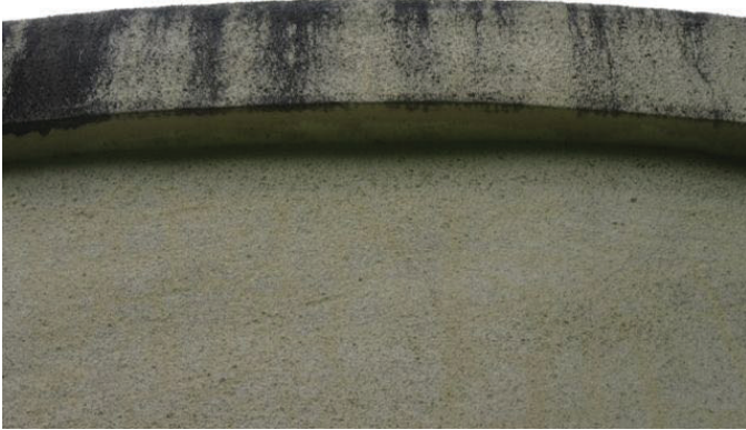
13 Exterior Wall With Mild Mildew
