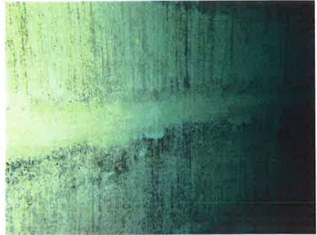
82 Interior Wall With Moderate To Heavy Staining
