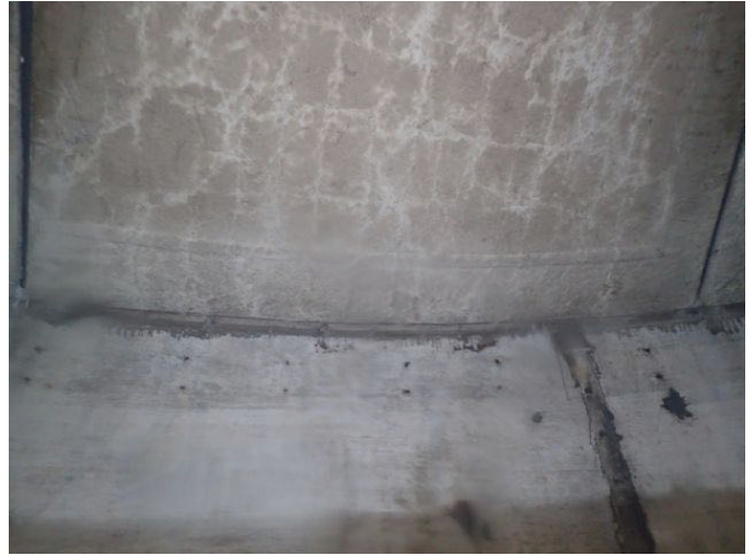
68 Interior Wall With Mild Staining
