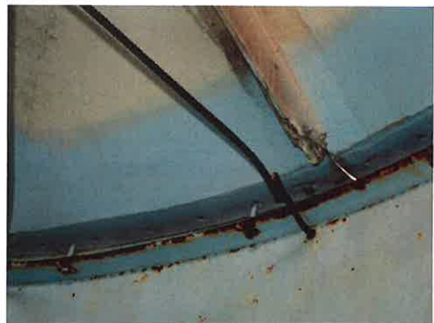
82 Overhead Spider Supports With Mild Surface Corrosion
