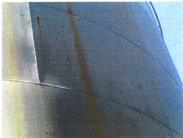
11 Exterior Wall With Coating Loss/Damage, Chalking Exposed Underlying Steel, Mild Surface Corrosion, Mildew And Corrosion Staining
