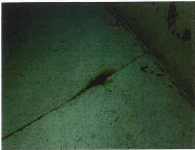
49 Floor With Ruptured Coating Blisters, Exposed Underlying Steel, Mild Surface Corrosion And Mild Staining
