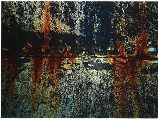
73 Interior Wall With Coating Loss (Nearing Expiration), Blotch Rusting, Exposed Underlying Steel, Moderate Surface Corrosion And Heavy Staining
