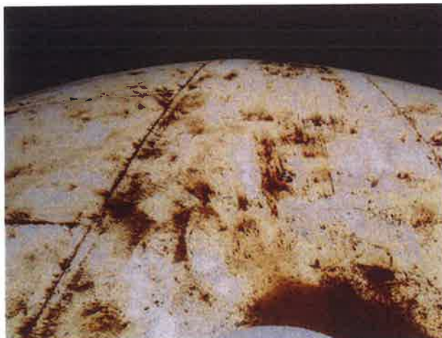
29 Roof With Coating Nearing Expiration, Exposed Primary Coating, Exposed Underlying Steel, Mild Surface Corrosion And Corrosion Staining
