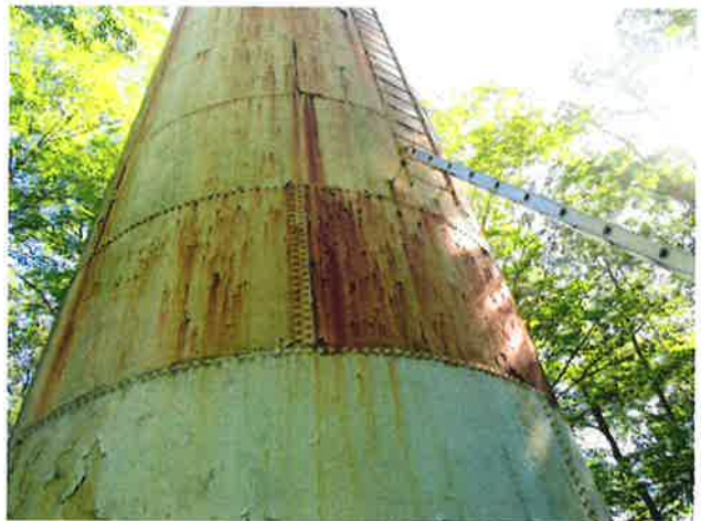
8 Exterior Wall With Expired Coating/Peeling, Exposed Underlying Steel, Blotch Rusting, Mild To Moderate Surface Corrosion, Corrosive Staining, Rust Staining And Mildew
