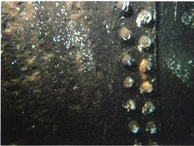
67 Interior Wall With Coating Loss (Nearing Expiration), Blotch Rusting, Exposed Underlying Steel, Moderate Surface Corrosion And Heavy Staining
