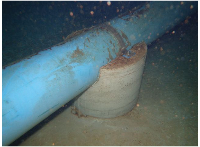
50 12" Inside Diameter P.V.C. Pipe Supported To The Tank Floor With Coating Loss/Blistering, Exposed Metal And Corrosion
