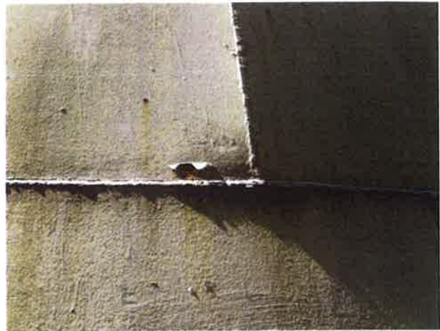
8 Exterior Wall With Coating Loss/Damage, Chalking Exposed Underlying Steel, Mild Surface Corrosion, Mildew And Corrosion Staining
