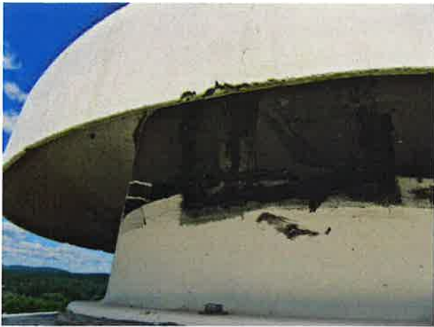
43 Vent Screen Found Torn
