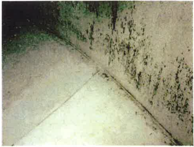
74 Interior Wall With Moderate To Heavy Staining
