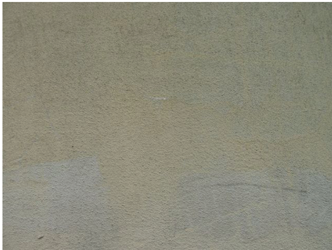
3 Exterior Wall With Coating Loss, Tight Shrinkage Cracks, Efflorescence And Mildew
