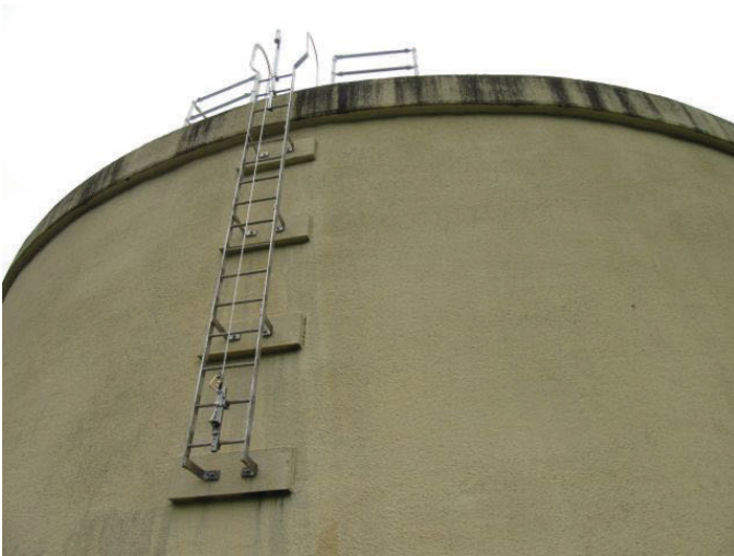
15 Ladder With A Fall Prevention Device
