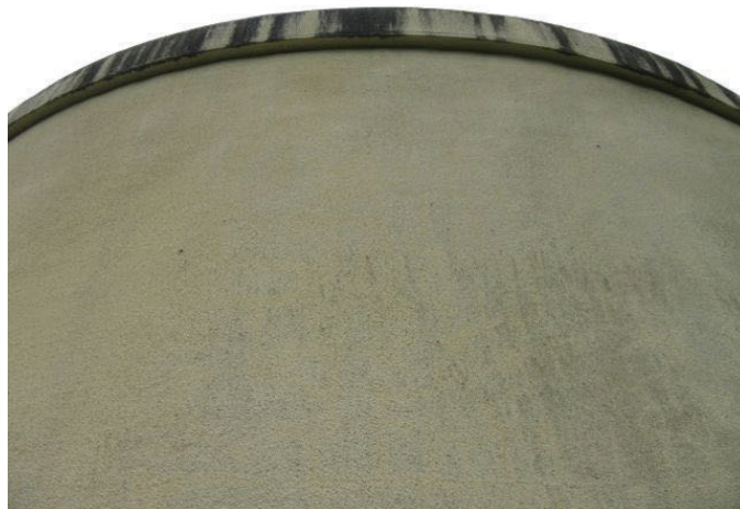
11 Exterior Wall With Mild Mildew
