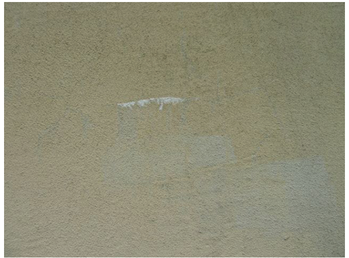
2 Exterior Wall With Coating Loss, Tight Shrinkage Cracks, Efflorescence And Mildew
