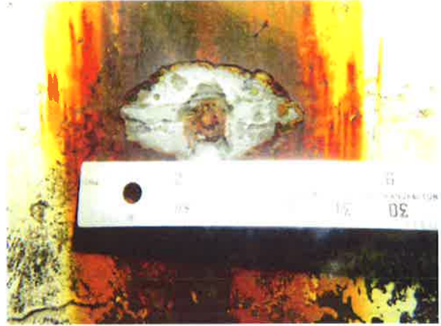
70 Interior Wall Welds With Coating Loss, Steel Fatigue (Pitting) And Moderate To Heavy Staining
