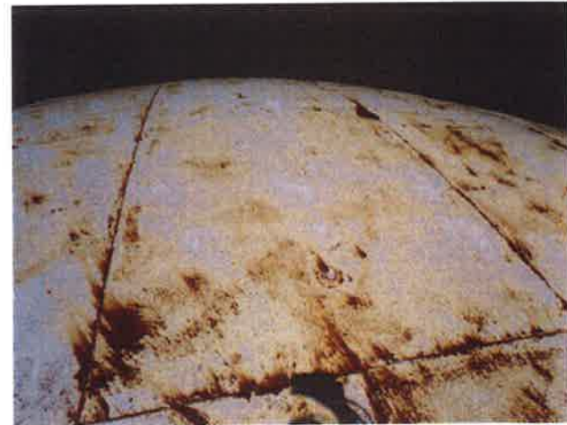
28 Roof With Coating Nearing Expiration, Exposed Primary Coating, Exposed Underlying Steel, Mild Surface Corrosion And Corrosion Staining
