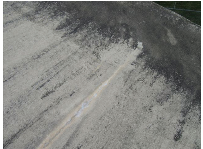
22 Roof Dome Concrete Filled Joints With Coating Loss, Tight Cracks And Mildew
