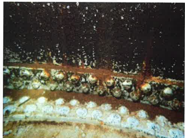
60 Interior Wall With Coating Loss (Nearing Expiration), Blotch Rusting, Exposed Underlying Steel, Moderate Surface Corrosion And Heavy Staining
