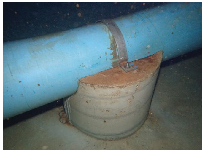
48 12" Inside Diameter P.V.C. Pipe Supported To The Tank Floor With Coating Loss/Blistering, Exposed Metal And Corrosion
