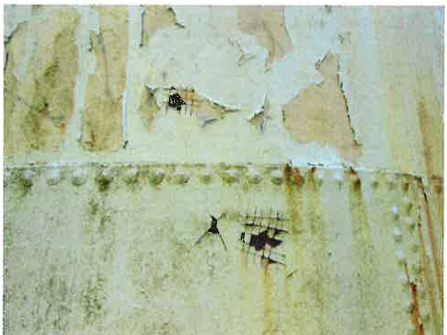
4 Exterior Wall With Expired Coating/Peeling, Cross Hatch Adhesion Test Causing Exposed Underlying Steel, Surface Corrosion And Mildew
