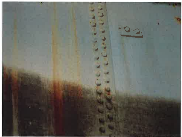
74 Interior Wall With Ruptured Coating Blisters, Exposed Underlying Steel, Mild To Moderate Surface Corrosion And Heavy Staining
