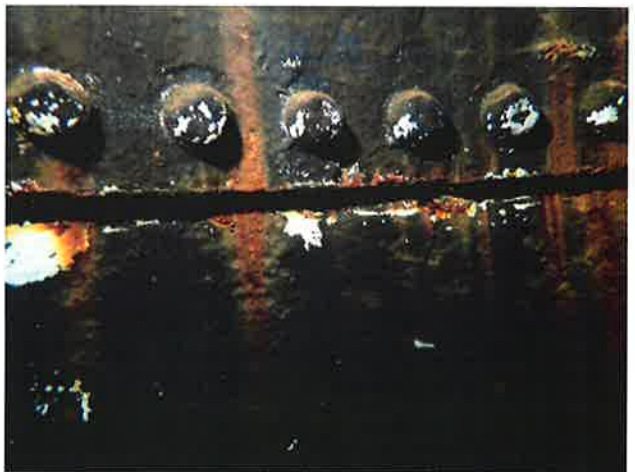
64 Interior Wall With Coating Loss (Nearing Expiration), Blotch Rusting, Exposed Underlying Steel, Moderate Surface Corrosion And Heavy Staining
