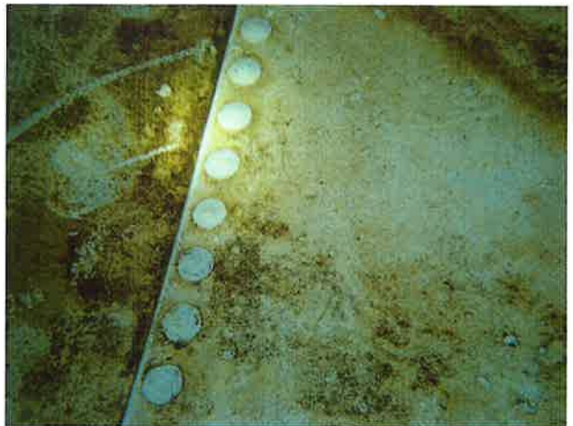
52 Floor With Mild Staining
