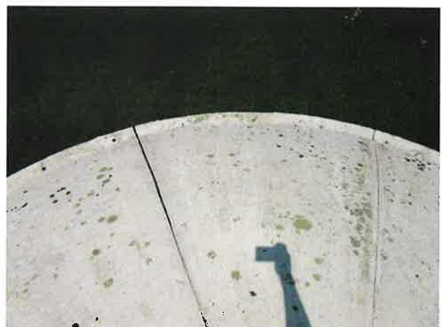
36 Roof Panel Joints Sealant Found Deteriorating
