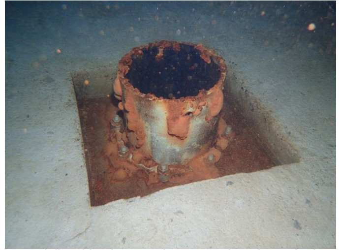
46 14" Inside Diameter Pipe Penetrating The Tank Floor Within A Deep Sump With Coating Loss/Blistering, Exposed Metal And Corrosion
