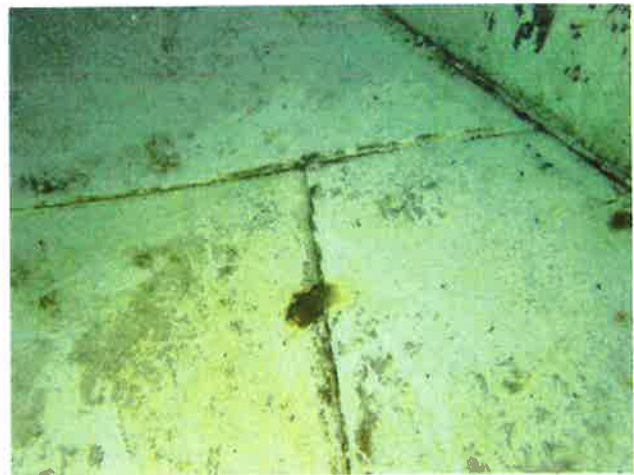
50 Floor With Ruptured Coating Blisters, Exposed Underlying Steel, Mild Surface Corrosion And Mild Staining
