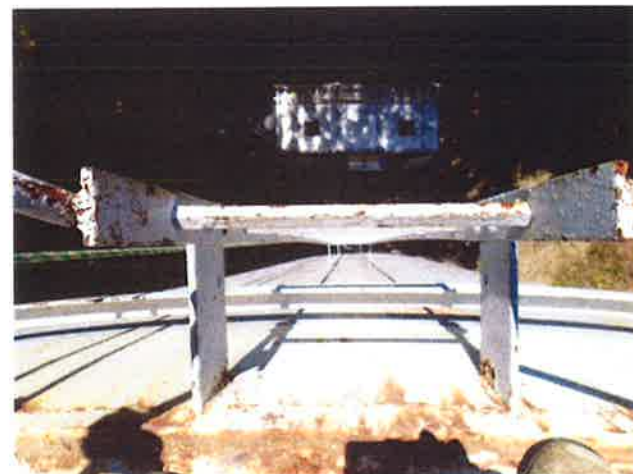
24 Roof Access Ladder With Coating Lifting/Peeling, Exposed Primary Coating, Exposed Underlying Steel And Mild Surface Corrosion
