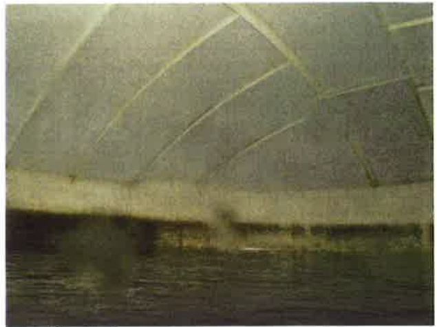
86 Overhead With Mild Blotch Rusting
