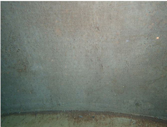
57 Interior Wall With Mild Staining
