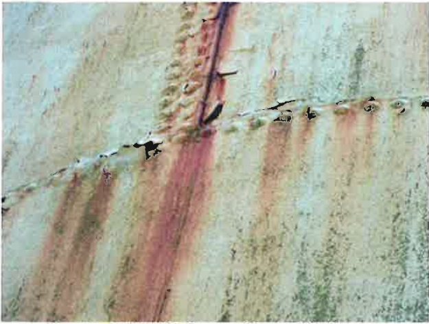
13 Exterior Wall With Expired Coating/Peeling, Exposed Underlying Steel, Blotch Rusting, Mild To Moderate Surface Corrosion, Corrosive Staining, Rust Staining And Mildew
