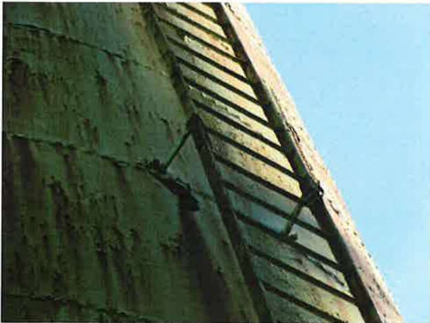
33 Ladder With Coating Loss (Nearing Expiration), Exposed Underlying Steel And Mild Corrosion
