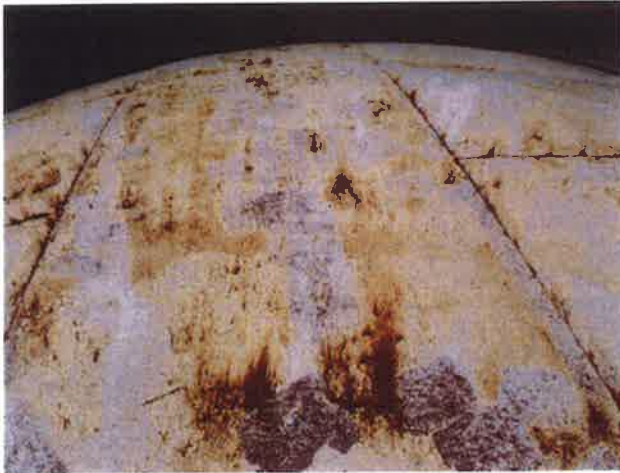
27 Roof With Coating Nearing Expiration, Exposed Primary Coating, Exposed Underlying Steel, Mild Surface Corrosion And Corrosion Staining
