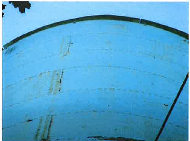
18 Exterior Wall With Expired Coating/Peeling, Exposed Underlying Steel, Blotch Rusting, Mild To Moderate Surface Corrosion, Corrosive Staining, Rust Staining And Mildew
