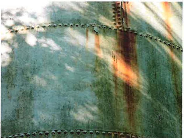
6 Exterior Wall With Expired Coating/Peeling, Exposed Underlying Steel, Blotch Rusting, Mild To Moderate Surface Corrosion, Corrosive Staining, Rust Staining And Mildew
