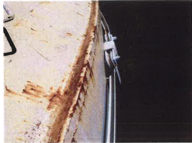
34 Roof With Coating Nearing Expiration, Exposed Primary Coating, Exposed Underlying Steel, Mild Surface Corrosion And Corrosion Staining
