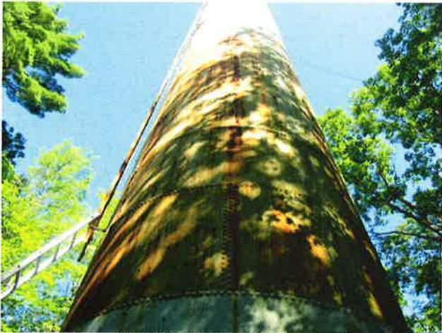
9 Exterior Wall With Expired Coating/Peeling, Exposed Underlying Steel, Blotch Rusting, Mild To Moderate Surface Corrosion, Corrosive Staining, Rust Staining And Mildew
