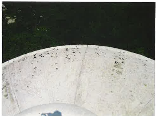
38 Roof Panel Joints Sealant Found Deteriorating
