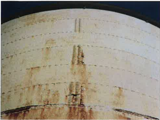
19 Exterior Wall With Expired Coating/Peeling, Exposed Underlying Steel, Blotch Rusting, Mild To Moderate Surface Corrosion, Corrosive Staining, Rust Staining And Mildew
