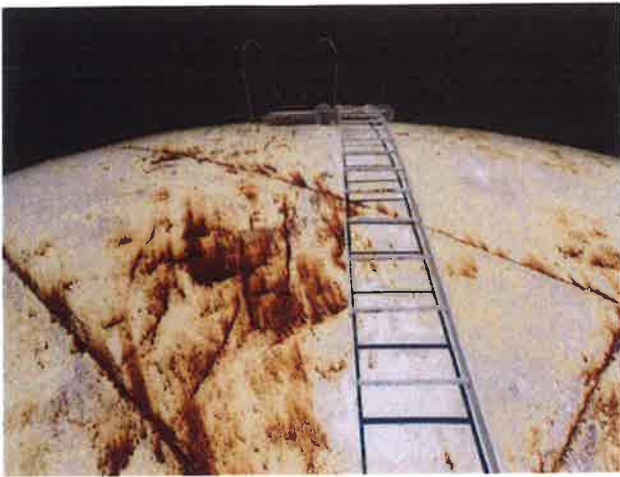
25 Vent Access Ladder With Coating Lifting/Peeling, Exposed Primary Coating, Exposed Underlying Steel And Mild Surface Corrosion
