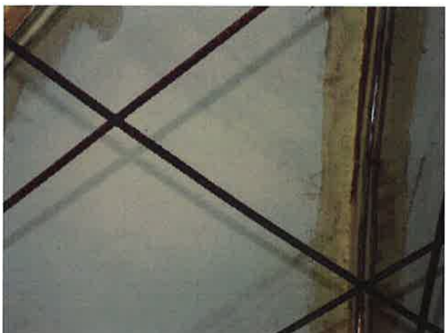
78 Overhead With Daylight Showing Through The Panel Joints
