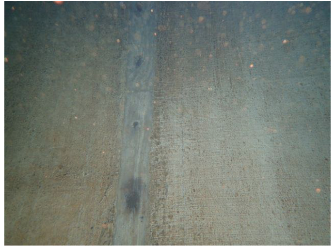
62 Interior Wall With Mild Staining
