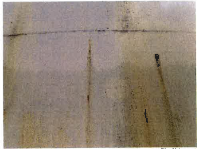
2 Exterior Wall With Coating Loss/Damage, Chalking Exposed Underlying Steel, Mild Surface Corrosion, Mildew And Corrosion Staining
