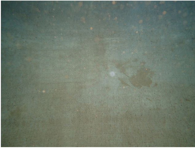
61 Interior Wall With Mild Staining
