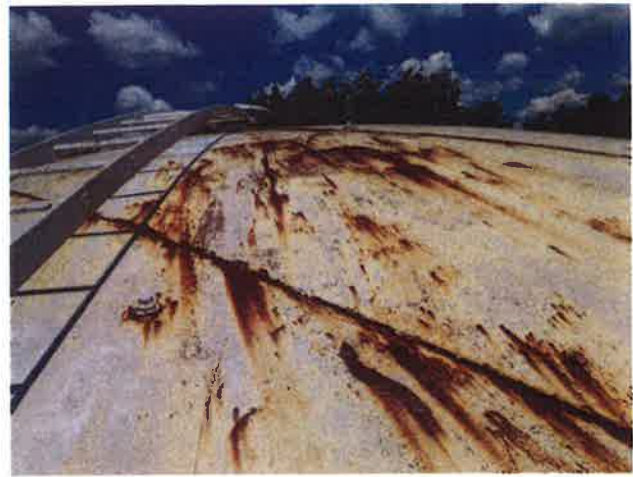
32 Roof With Coating Nearing Expiration, Exposed Primary Coating, Exposed Underlying Steel, Mild Surface Corrosion And Corrosion Staining
