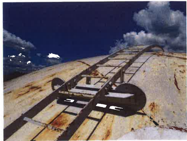
26 Vent Access Ladder With Coating Lifting/Peeling, Exposed Primary Coating, Exposed Underlying Steel And Mild Surface Corrosion
