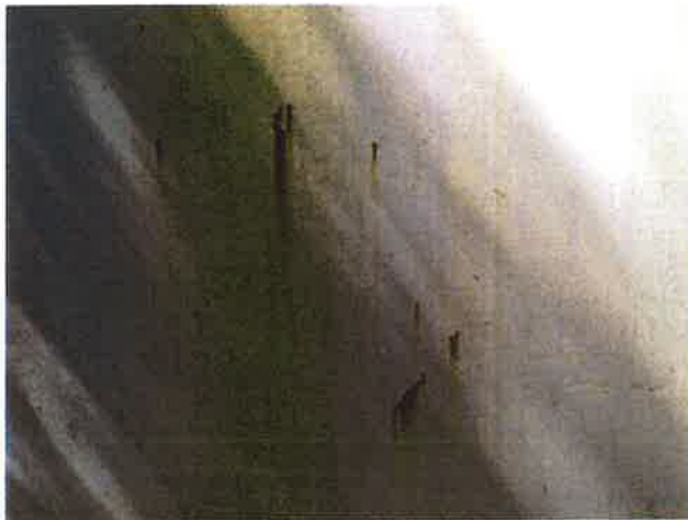
9 Exterior Wall With Coating Loss/Damage, Chalking Exposed Underlying Steel, Mild Surface Corrosion, Mildew And Corrosion Staining
