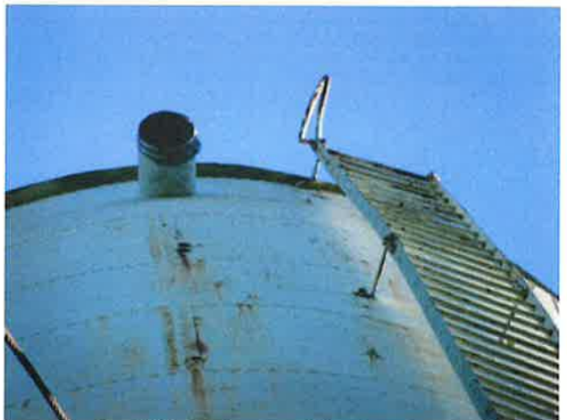
34 Ladder With Coating Loss (Nearing Expiration), Exposed Underlying Steel And Mild Corrosion
