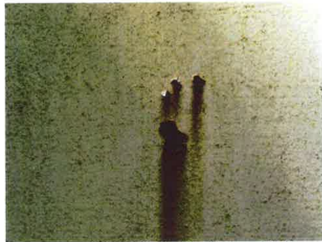
10 Exterior Wall With Coating Loss/Damage, Chalking Exposed Underlying Steel, Mild Surface Corrosion, Mildew And Corrosion Staining
