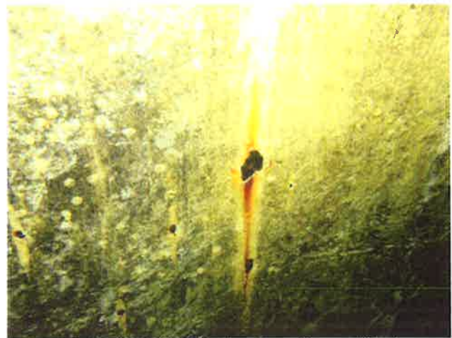
64 Interior Wall With Coating Loss, Exposed Steel, Surface Corrosion And Moderate To Heavy Staining
