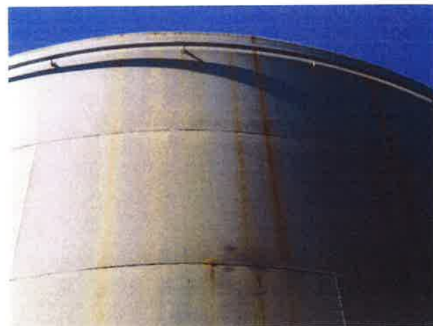
12 Exterior Wall With Coating Loss/Damage, Chalking Exposed Underlying Steel, Mild Surface Corrosion, Mildew And Corrosion Staining
