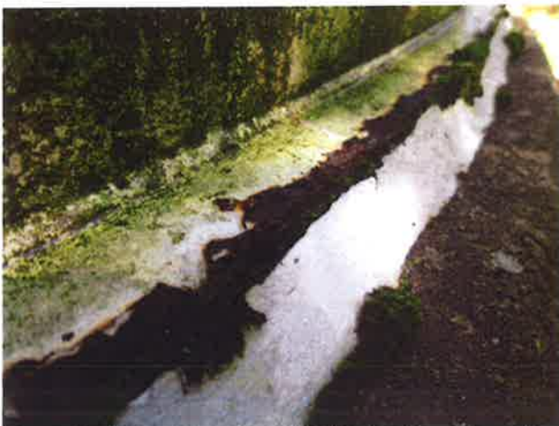
15 Steel Floor Extension With Coating Loss, Exposed Steel, Mild To Moderate Surface Corrosion And Mildew
