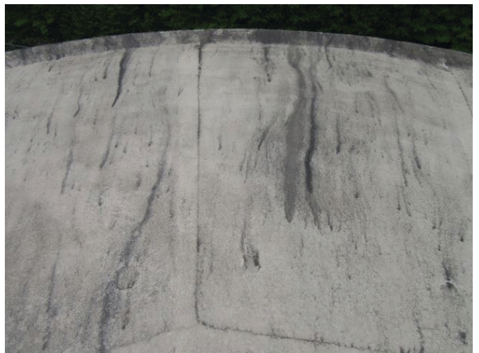
18 Roof Dome Concrete Filled Joints With Coating Loss, Tight Cracks And Mildew
