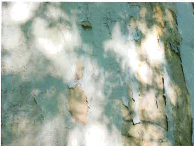
11 Exterior Wall With Expired Coating/Peeling, Exposed Underlying Steel, Blotch Rusting, Mild To Moderate Surface Corrosion, Corrosive Staining, Rust Staining And Mildew
