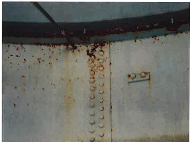
76 Interior Wall With Ruptured Coating Blisters, Exposed Underlying Steel, Mild To Moderate Surface Corrosion And Heavy Staining
