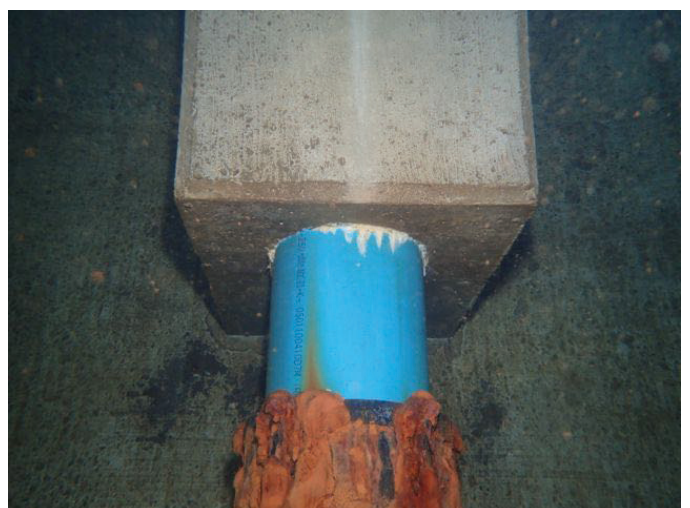
84 Overflow Pipe Extending Through A Coupling/ Penetrating A Concrete Box With Expired Coating And Exposed Underlying Steel
