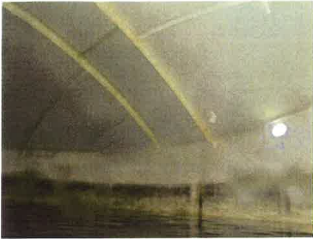
85 Interior Wall With Moderate To Heavy Staining
