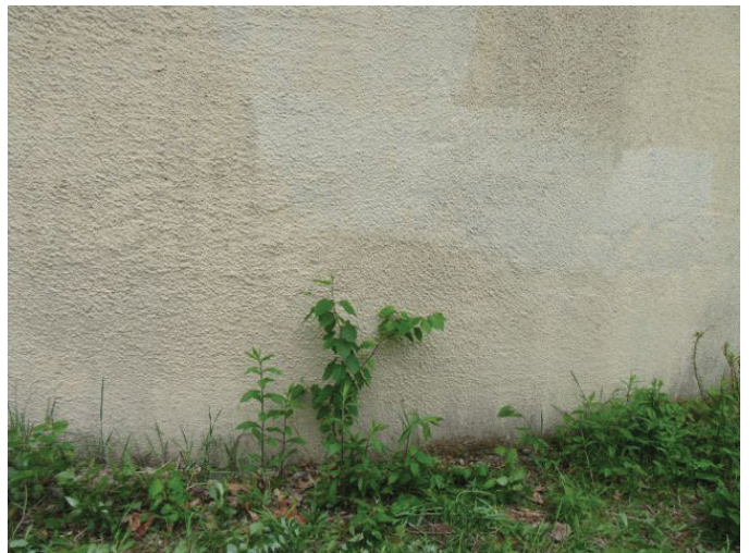
6 Exterior Wall With Mild Mildew
