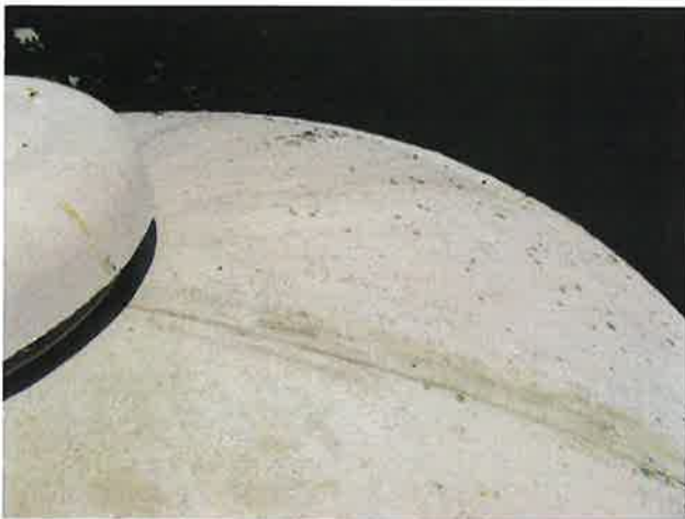
39 Roof Panel Joints Sealant Found Deteriorating
