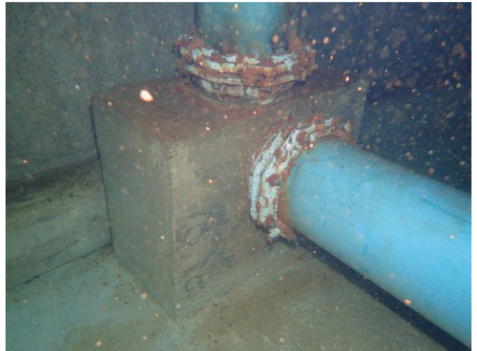
52 12" Inside Diameter Pipe Elbow Encased In A Concrete Thrust Block
