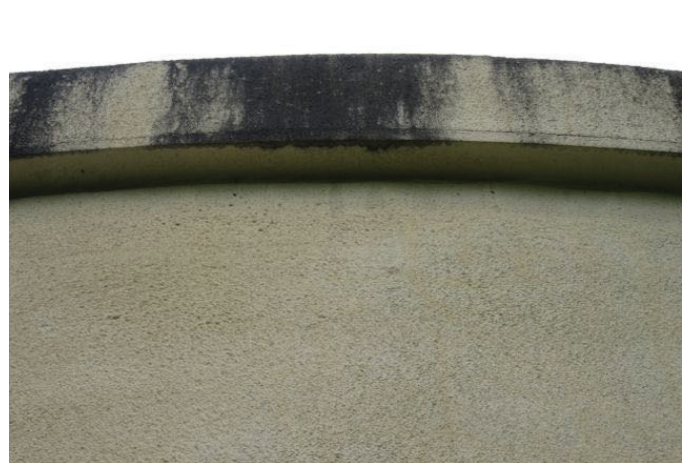
12 Exterior Wall With Mild Mildew
