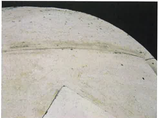
40 Roof Panel Joints Sealant Found Deteriorating
