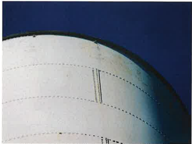
20 Exterior Wall With Expired Coating/Peeling, Exposed Underlying Steel, Blotch Rusting, Mild To Moderate Surface Corrosion, Corrosive Staining, Rust Staining And Mildew
