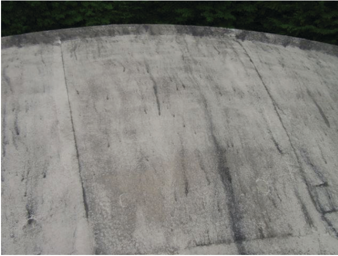
19 Roof Dome Concrete Filled Joints With Coating Loss, Tight Cracks And Mildew
