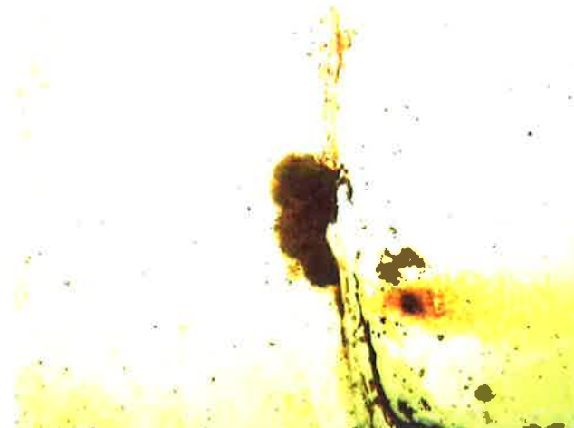
54 Floor With Ruptured Coating Blisters, Exposed Underlying Steel, Mild Surface Corrosion And Mild Staining
