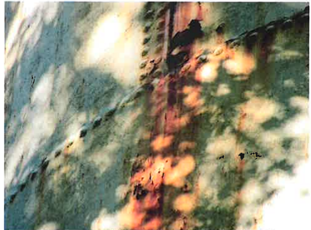
16 Exterior Wall With Expired Coating/Peeling, Exposed Underlying Steel, Blotch Rusting, Mild To Moderate Surface Corrosion, Corrosive Staining, Rust Staining And Mildew
