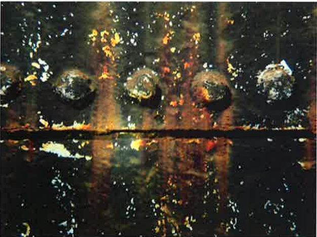
69 Interior Wall With Coating Loss (Nearing Expiration), Blotch Rusting, Exposed Underlying Steel, Moderate Surface Corrosion And Heavy Staining
