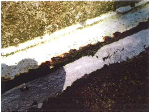
21 Concrete Foundation - Tank Base To Wall Junction With Sealant Degrading Due To Weathering
