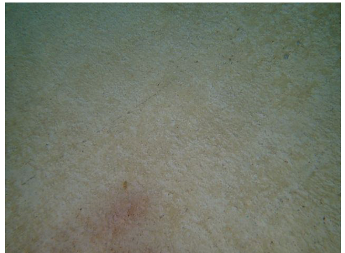
36 Floor With Mild Staining
