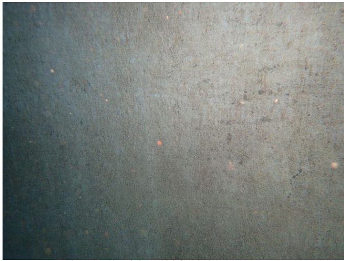
63 Interior Wall With Mild Staining
