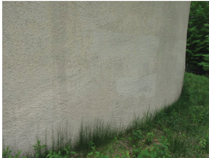
9 Exterior Wall With Mild Mildew
