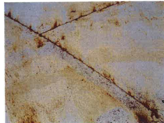
30 Roof With Coating Nearing Expiration, Exposed Primary Coating, Exposed Underlying Steel, Mild Surface Corrosion And Corrosion Staining
