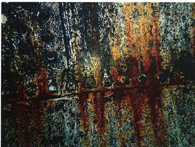
71 Interior Wall With Coating Loss (Nearing Expiration), Blotch Rusting, Exposed Underlying Steel, Moderate Surface Corrosion And Heavy Staining
