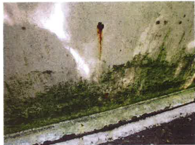
16 Steel Floor Extension With Coating Loss, Exposed Steel, Mild To Moderate Surface Corrosion And Mildew
