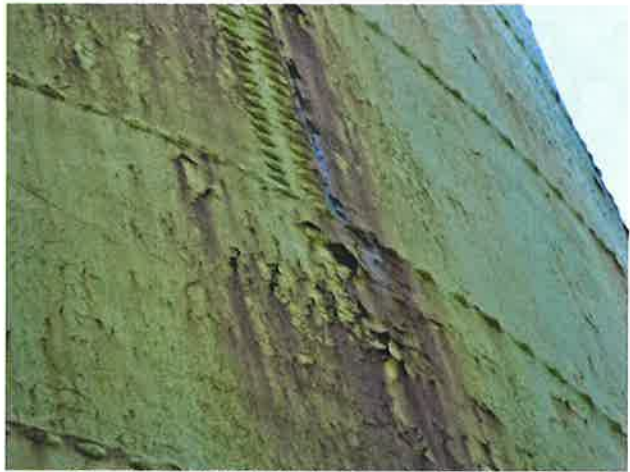
14 Exterior Wall With Expired Coating/Peeling, Exposed Underlying Steel, Blotch Rusting, Mild To Moderate Surface Corrosion, Corrosive Staining, Rust Staining And Mildew
