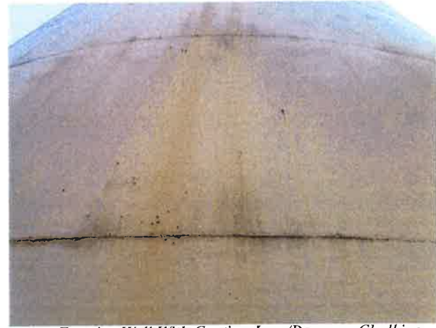
4 Exterior Wall With Coating Loss/Damage, Chalking Exposed Underlying Steel, Mild Surface Corrosion, Mildew And Corrosion Staining
