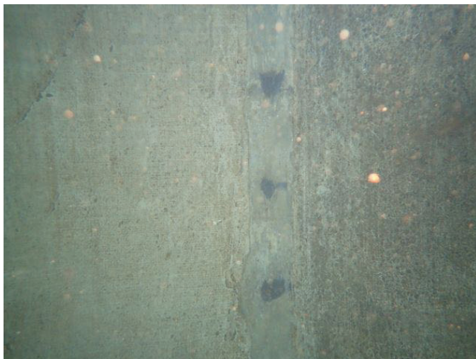
65 Interior Wall With Mild Staining
