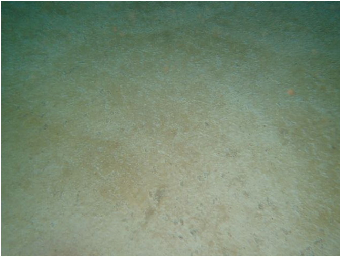
37 Floor With Mild Staining
