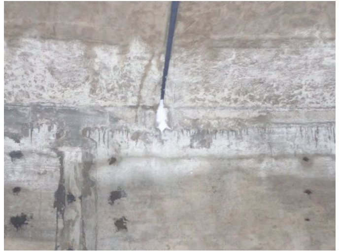
80 Overhead With Panel Joints/Edges With Efflorescence
