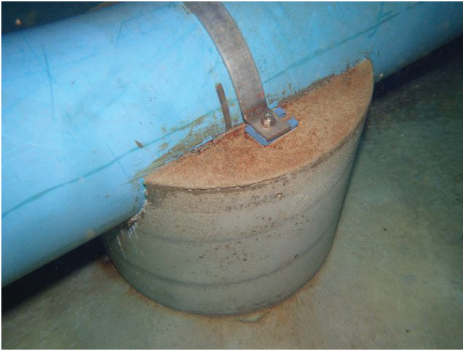
49 12" Inside Diameter P.V.C. Pipe Supported To The Tank Floor With Coating Loss/Blistering, Exposed Metal And Corrosion
