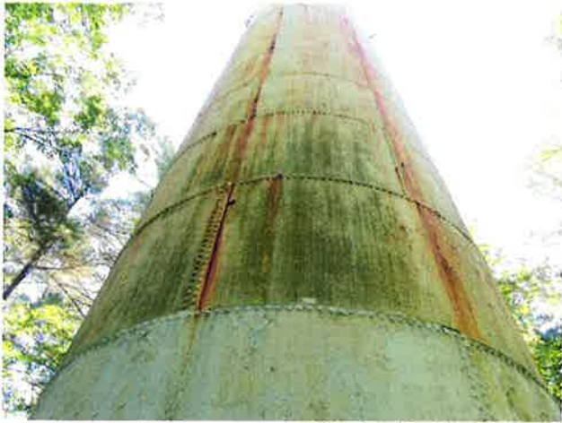
7 Exterior Wall With Expired Coating/Peeling, Exposed Underlying Steel, Blotch Rusting, Mild To Moderate Surface Corrosion, Corrosive Staining, Rust Staining And Mildew
