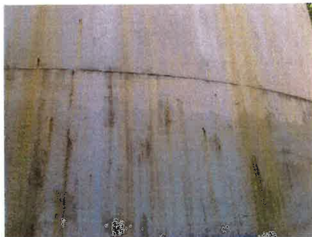
5 Exterior Wall With Coating Loss/Damage, Chalking Exposed Underlying Steel, Mild Surface Corrosion, Mildew And Corrosion Staining
