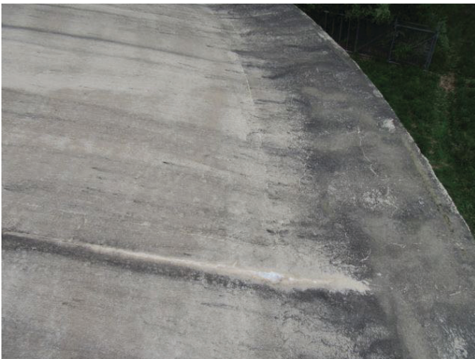
23 Roof Dome Concrete Filled Joints With Coating Loss, Tight Cracks And Mildew
