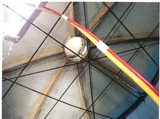
80 Overhead With Daylight Showing Through The Panel Joints
