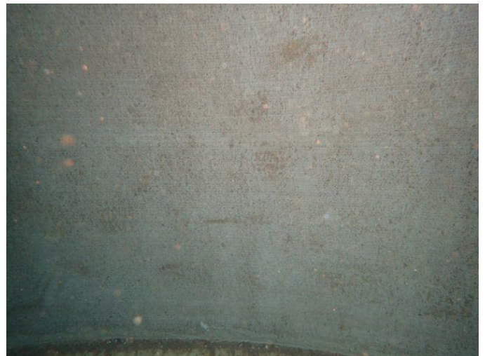
58 Interior Wall With Mild Staining
