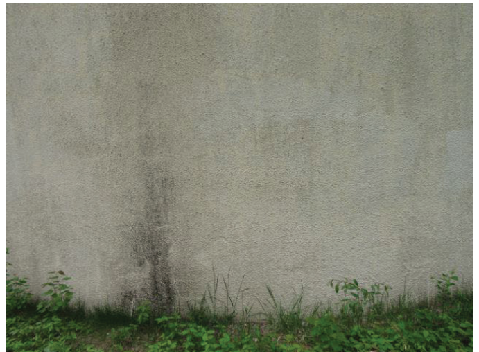
10 Exterior Wall With Mild Mildew
