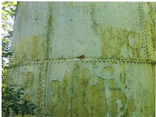
2 Exterior Wall With Expired Coating/Peeling, Exposed Underlying Primary Coating, Rust Staining And Mildew
