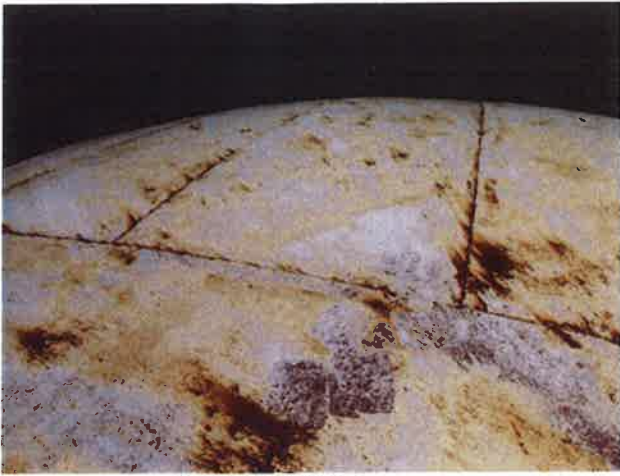
31 Roof With Coating Nearing Expiration, Exposed Primary Coating, Exposed Underlying Steel, Mild Surface Corrosion And Corrosion Staining
