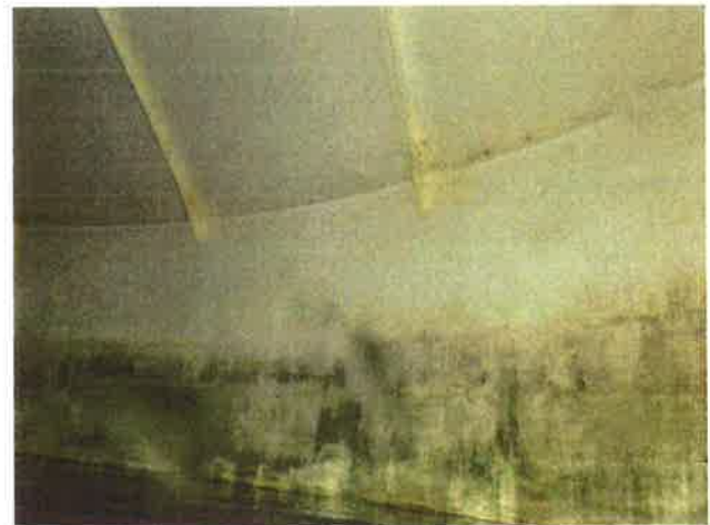
84 Interior Wall With Moderate To Heavy Staining
