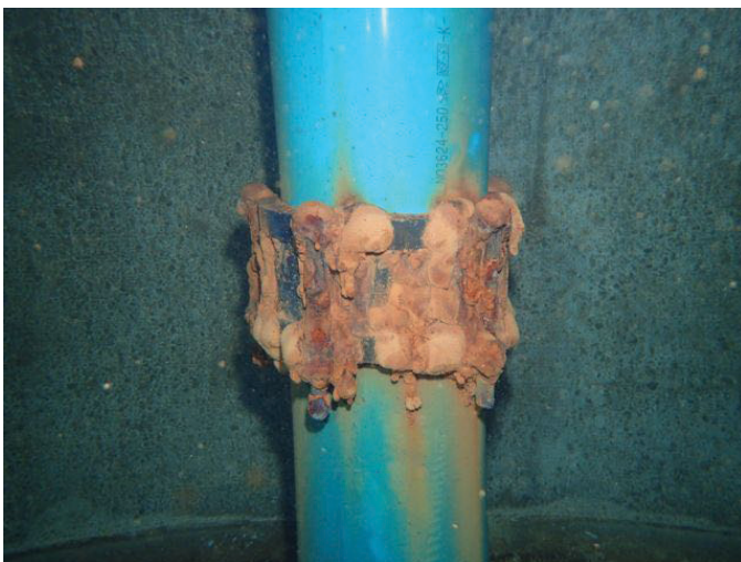
83 Overflow Pipe Extending Through A Coupling With Expired Coating And Exposed Underlying Metal
