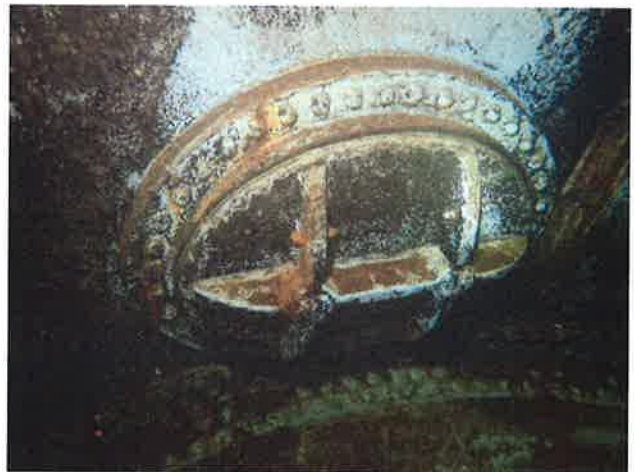
56 Manway Rivets With Coating Loss And Mild Corrosion
