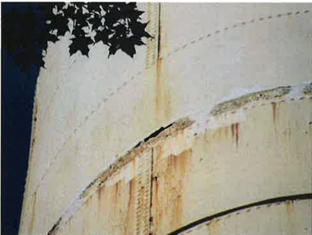
17 Exterior Wall With Expired Coating/Peeling, Exposed Underlying Steel, Blotch Rusting, Mild To Moderate Surface Corrosion, Corrosive Staining, Rust Staining And Mildew
