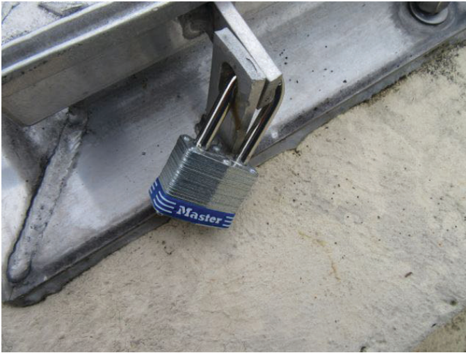
31 Secure Access Hatch
