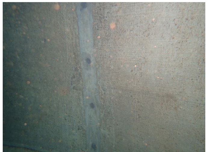
60 Interior Wall With Mild Staining
