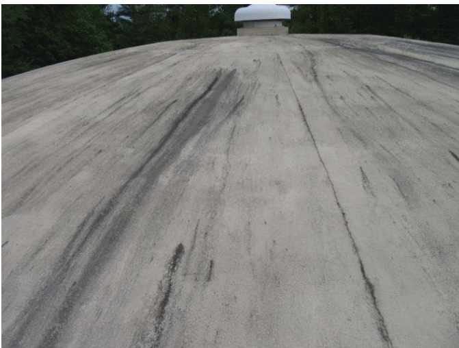
17 Roof Dome With Mildew
