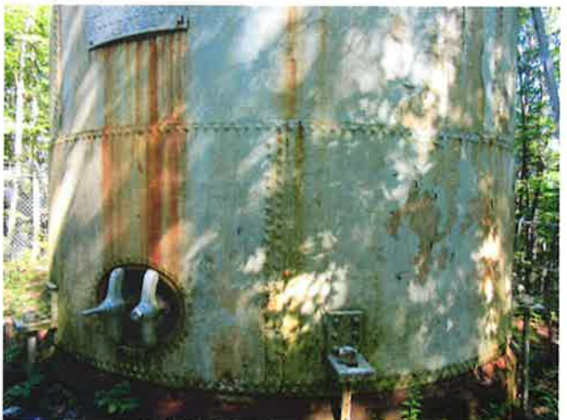
10 Exterior Wall With Expired Coating/Peeling, Exposed Underlying Steel, Blotch Rusting, Mild To Moderate Surface Corrosion, Corrosive Staining, Rust Staining And Mildew
