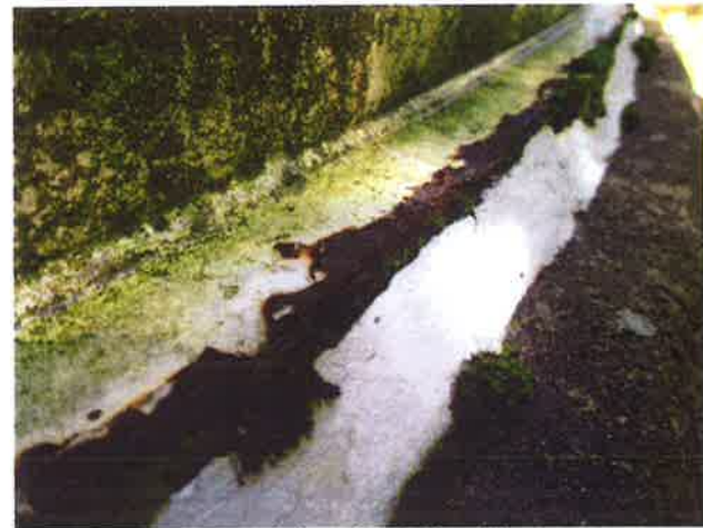
22 Concrete Foundation - Tank Base To Wall Junction With Sealant Degrading Due To Weathering
