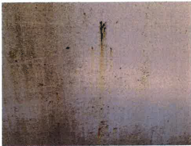
3 Exterior Wall With Coating Loss/Damage, Chalking Exposed Underlying Steel, Mild Surface Corrosion, Mildew And Corrosion Staining
