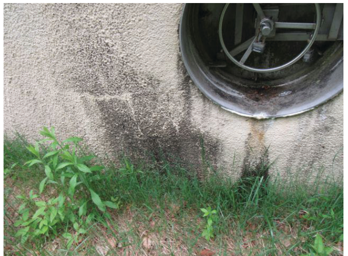
4 Exterior Wall With Coating Loss, Tight Shrinkage Cracks, Efflorescence And Mildew
