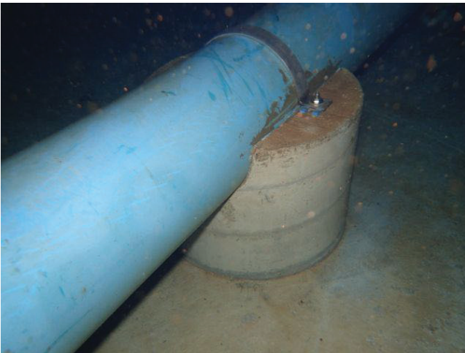
51 12" Inside Diameter P.V.C. Pipe Supported To The Tank Floor With Coating Loss/Blistering, Exposed Metal And Corrosion
