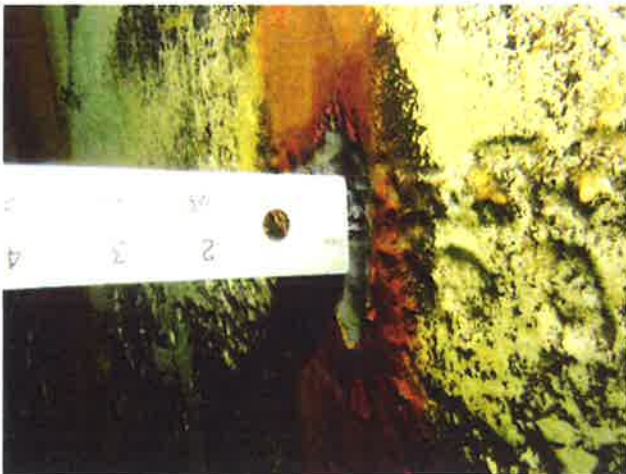
71 Interior Wall Welds With Coating Loss, Steel Fatigue (Pitting) And Moderate To Heavy Staining
