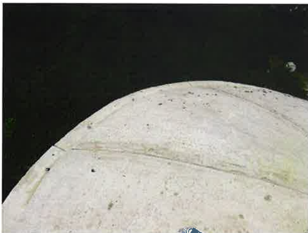
41 Roof Panel Joints Sealant Found Deteriorating
