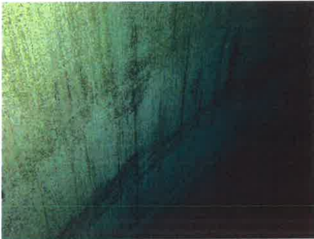
81 Interior Wall With Moderate To Heavy Staining
