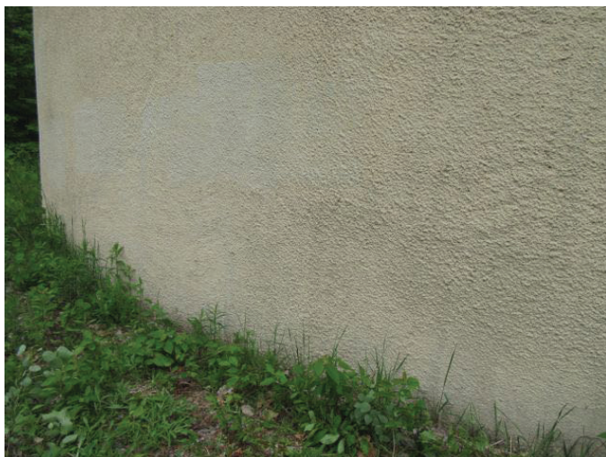
5 Exterior Wall With Mild Mildew
