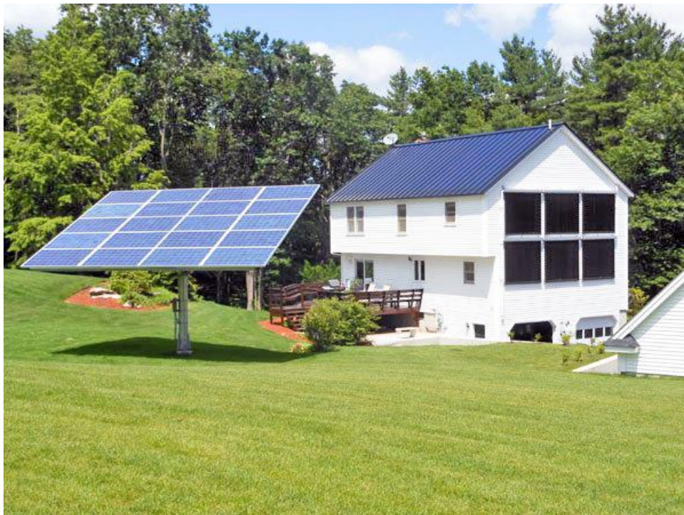
Tracker Mounted Residential System: Courtesy Revision Energy
